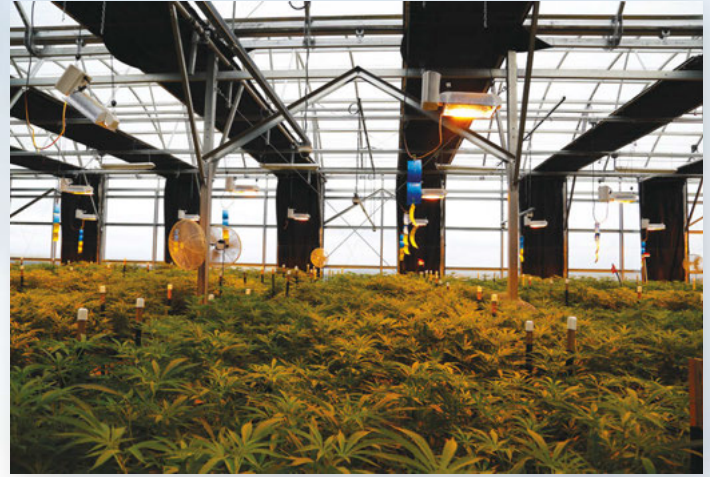
Above: An automated light deprivation system in use. Background Image: This operation has dialed back its artificial lighting needs by using natural sunlight.
